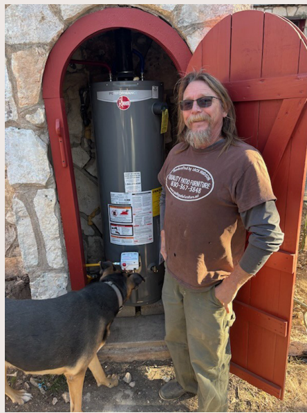
Jack Hudson stands beside the new electric water heater purchased by OGT to replace the previous one that was destroyed by the flood.
