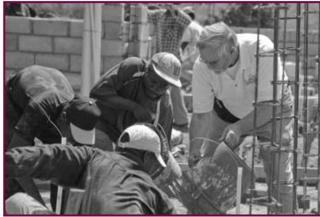
Rev. Glenn Merritt (right) helps pour concrete at a construction site in Haiti. He will report on Haiti relief efforts at the September convention in Norfolk.
