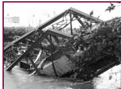
Railroad bridge at Cedar Rapids, Iowa, was destroyed by water 20-feet over flood stage.
