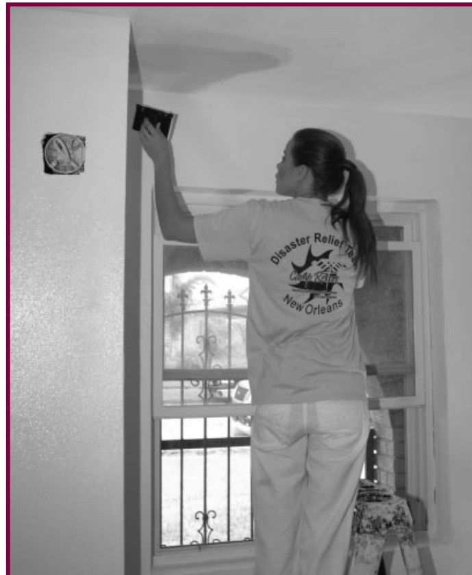
Katie helped paint a room in Chiquita Day's home with other Camp Restore and Camp Biloxi volunteers. Miss Day is living with relatives while the restoration continues.
